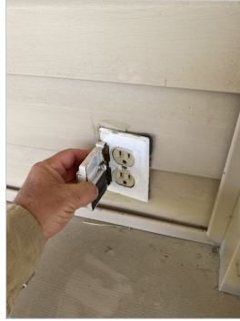
Not GFCI Protected
