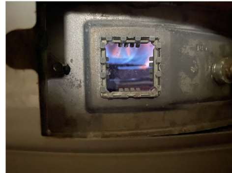
Water Heater Flame
