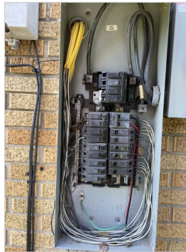
Outside Main Panel
