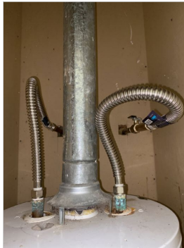
Hose Connections not Dielectric
