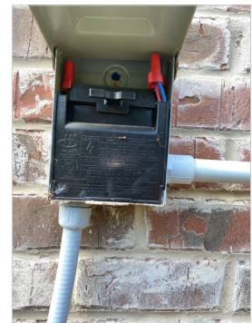
Improper device for electrical connection at condenser unit.
