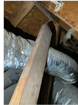
HVAC power switch in attic is not fastened on either end.
