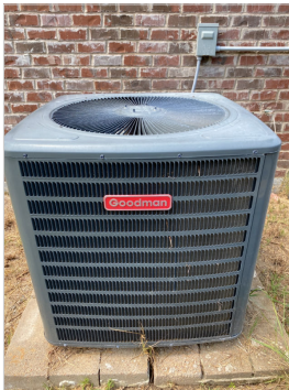
Goodman Condenser Unit
