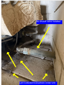
No gas shutoff valve installed.
