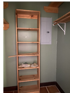
Insufficient clearance and next to clothes rack.
