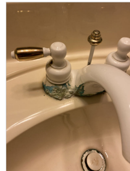
Upstairs Bath faucet leaking and corroded.
