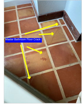
Master Bath: Tile had hair line crack.
