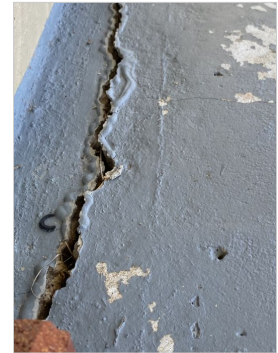
Crack along the wall.
