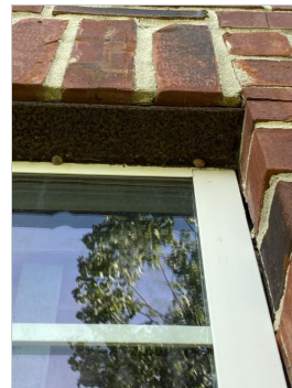
No seal. Lintel rusted.
