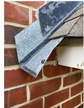
Carport wall flashing extended for drainage. Gutters should be properly installed.
