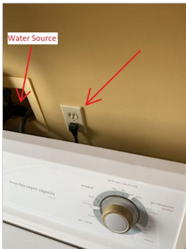
Washer receptacle not GFCI protected.
