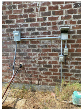
Condenser and Septic Tank Blower Disconnect.
