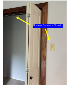
Upstairs Bedroom Closet: Light not functioning.
