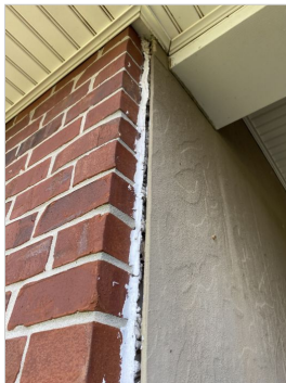
Carport wall should be resealed to brick.
