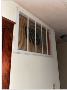
Return Upstairs: No filter was present.
