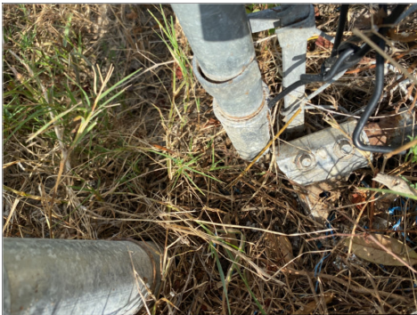
Gate fitting is cracked.
