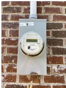
Utility Service Meter
