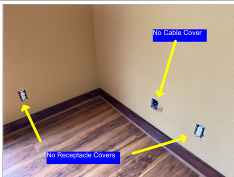
Electrical devices need covers. Some receptacles need replacement due to excess paint.
