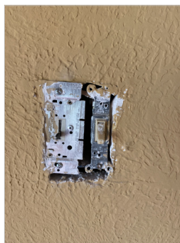
Dining room switch needs cover.
