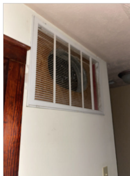
Return Upstairs: No filter was present.
