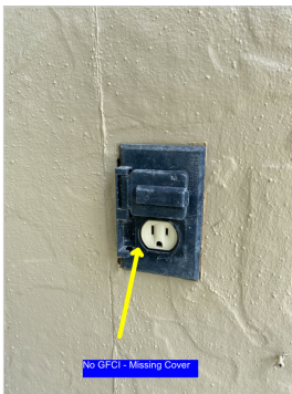
Front Patio: Not GFCI protected and missing weatherproof safety cover
