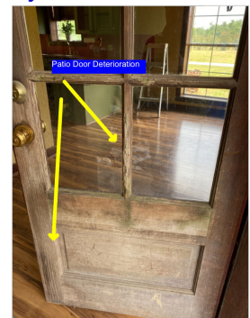
Rear patio door was deteriorated.
