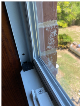
Recommend safety lock to prevent fall hazard.
