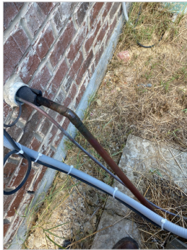
Condenser suction line not insulated.
