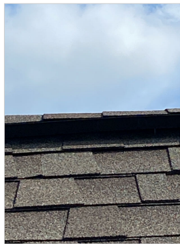
Ridge vent should be fastened to prevent pest and moisture intrusion to attic.
