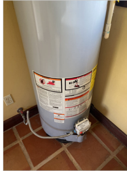
WATER HEATER Drip Pan
