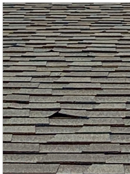
Shingles not bonded
