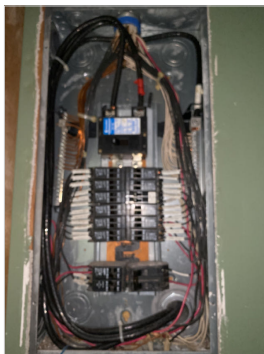
Electrical Panel was in satisfactory condition.
