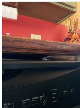
Dishwasher needs to be properly supported to countertop.
