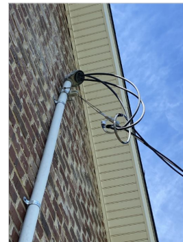
Utility Service Cable
