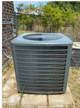
Goodman Condenser Unit
