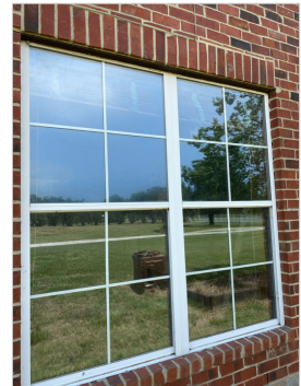
Windows not sealed.
