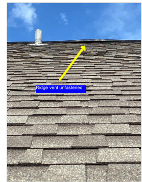
Ridge vent is unfastened in several areas.
