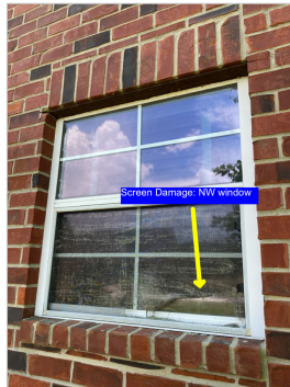
Northwest Window: Screen damage.
