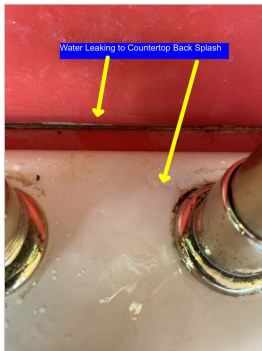
Kitchen faucet base leaking. Signs of water damage appeared in cabinet below sink.
