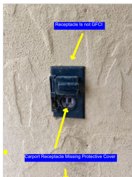
Carport receptacle is not GFCI protected and missing a safety cover.
