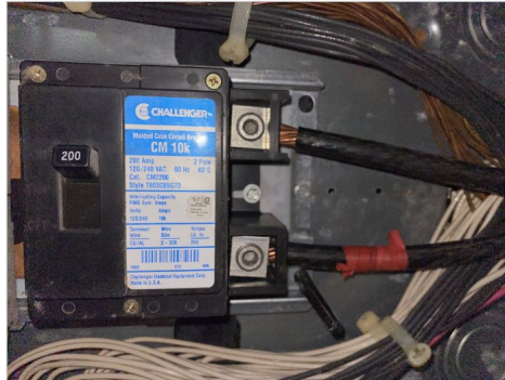
Service Panel Main Breaker, Challenger 200A
