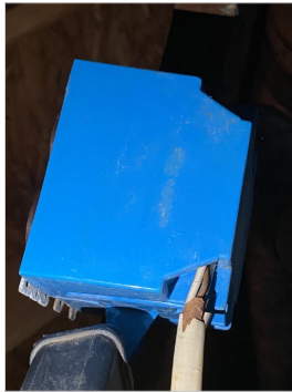
Missing cover for Indoor HVAC Unit power switch/receptacle.
