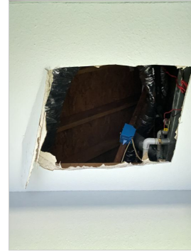
No permanent attic access.
