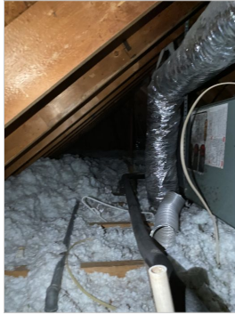
No Work Platform, Limited Access
