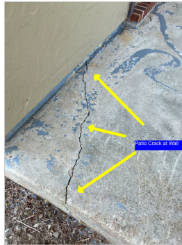
Front Patio: North end of lateral crack.
