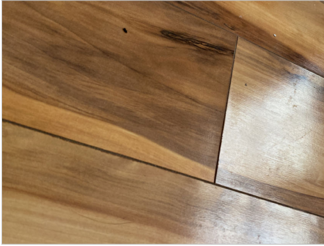
Kitchen laminate flooring buckling due to water exposure.
