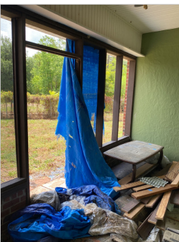
Back patio screens were missing. Excessive debris.
