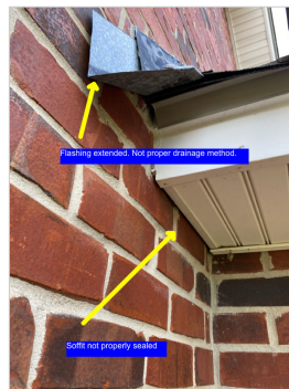
Soffit should be sealed to prevent pest intrusion.
