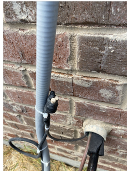
Exposed wiring connection for thermostat.
