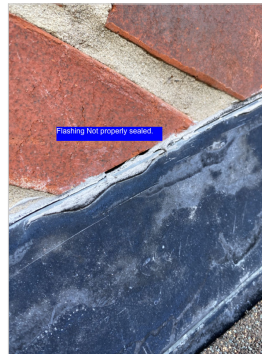
Carport wall flashing sealant should be removed and replaced with fresh sealant.
