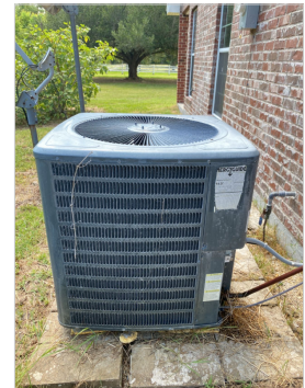
Goodman Condenser Unit
