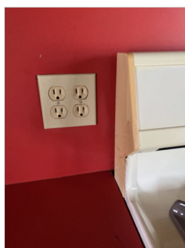
Kitchen receptacles are not GFCI protected.
