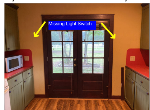
Kitchen light switch should be located at door entry.
