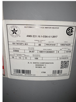
Water Heater Data
