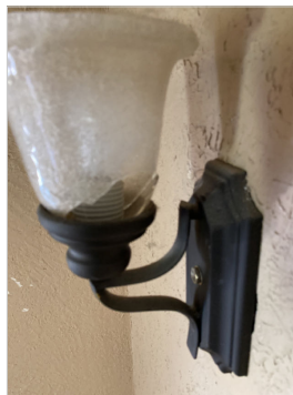
Stairway fixture glass shade cracked at base.
