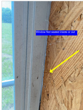
Window not sealed properly outside or inside.
