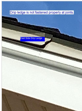
Drip Ledge Joints not Fastened Properly
