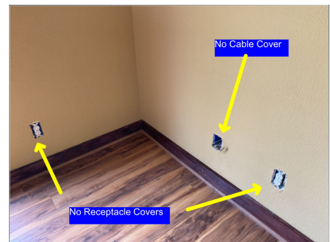
Electrical devices need covers. Some receptacles need replacement due to excess paint.
