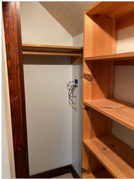
Wiring in upstairs bedroom-2 closet needs to be covered properly.
