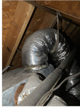
Air Duct Rust
