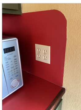
Kitchen receptacles are not GFCI protected.
