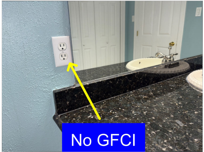
No GFCI in upstairs bathroom.
