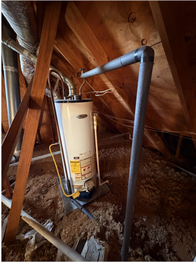
Water lines were not supported sufficiently.
