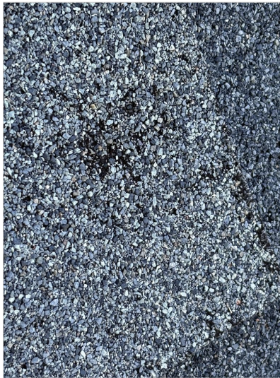
Area with granules removed from shingles.
