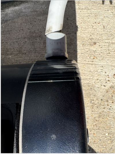
PVC conduit was disconnected from the adapter fitting at the pump.
