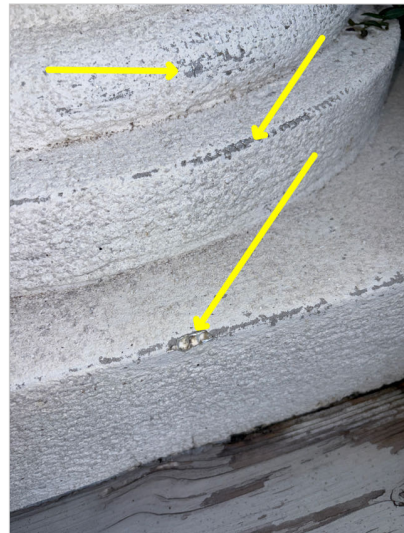
Column base deterioration.
