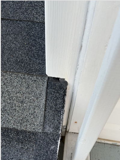
Insufficient flashing and sealant located at end of balcony.
