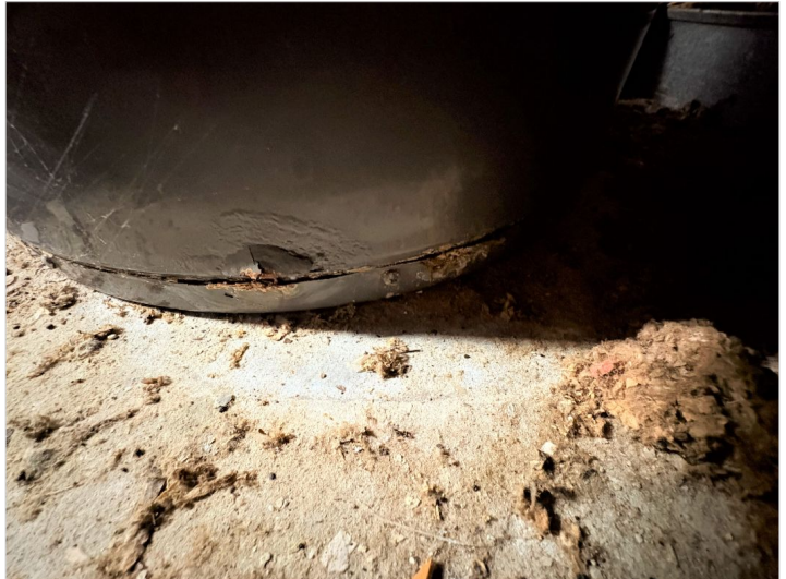
Tank was showing signs of rust.
