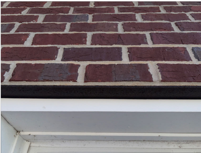
Sealant needed above window.
