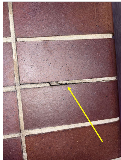
Coping tiles need mortar sealant applied to prevent moisture intrusion that can cause settlement or heaving of perimeter slab.
