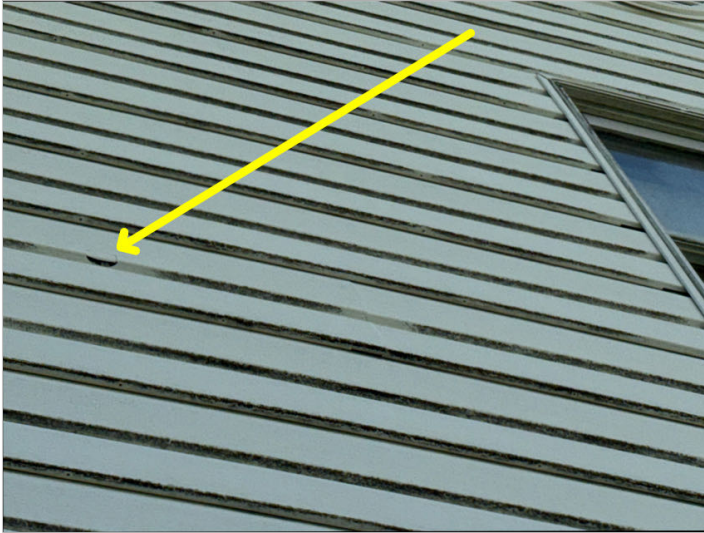
Small hole in vinyl siding.
