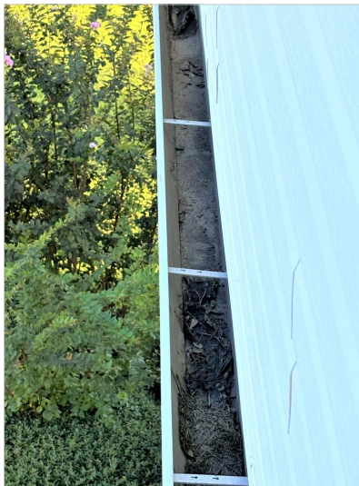
Debris was inside gutter located at rear-right side of home above patio.
