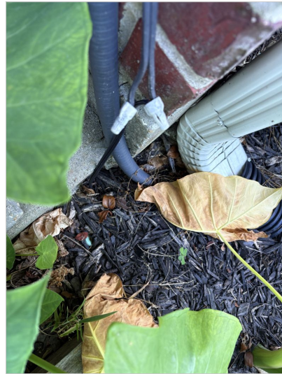
Circuit for HVAC timer was spliced without the use of an electrical termination box.
