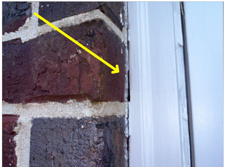
Rear garage entry door frame to brick sealant deterioration.
