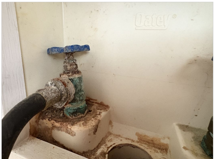
Washing machine hose bib significantly corroded.
