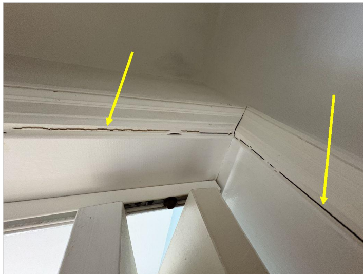
Upstairs closet door trim needs to be resealed.
