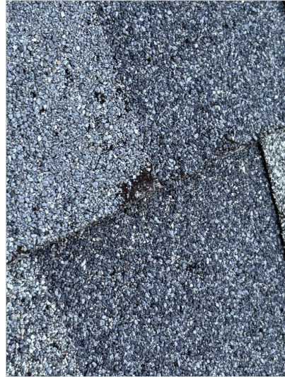
Area with granules removed from shingles.
