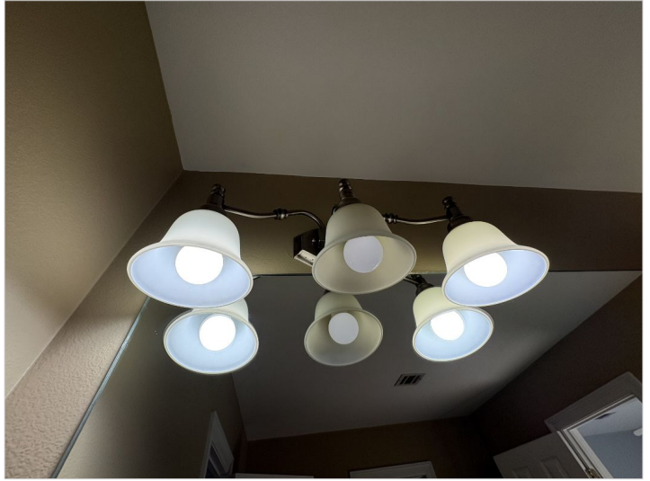
Upstairs bathroom vanity light bulb did not illuminate.
