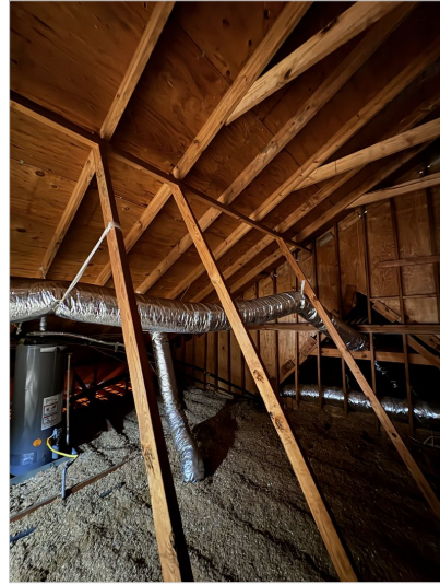
Support boards not strengthened by T-Back board.
