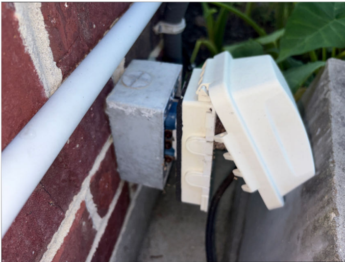
Sewer system blower receptacle not secured in electrical device box.
