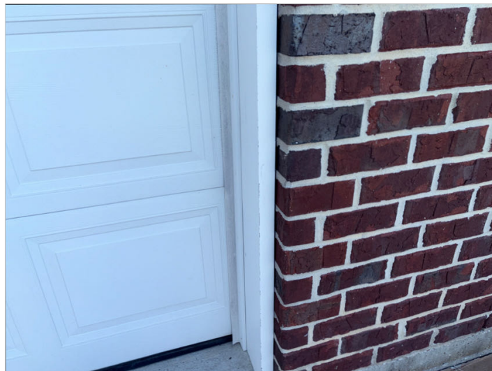
No sealant was applied between support board and brick. Located at pool area garage roll up door.
