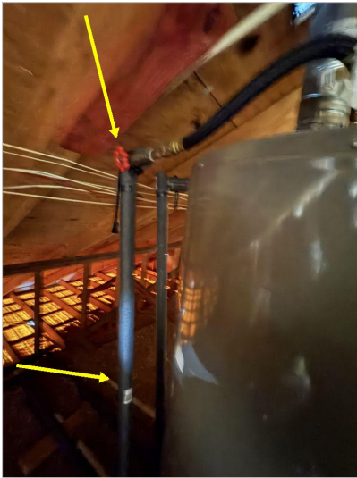
Water lines not supported.
