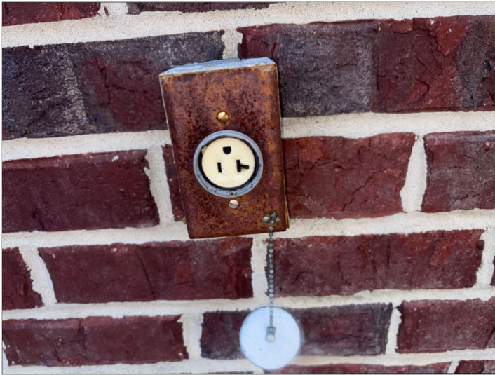
Rear patio receptacle was not ground fault circuit interrupting type.
