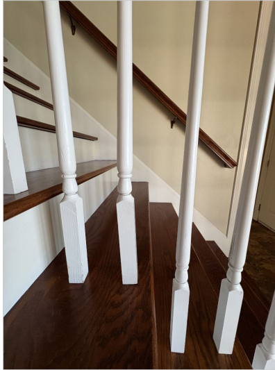
The stairs had a baluster that was broken.
