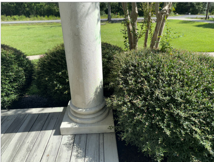
Vegetation in contact with deck.
