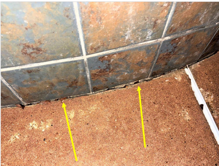
Close-up of hot tub to slab joint needing sealant.
