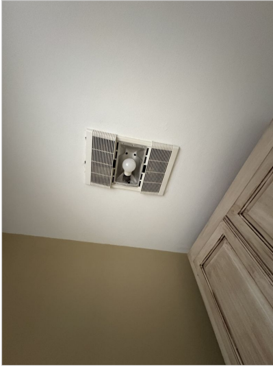
Upstairs bathroom lighting lens was missing.
