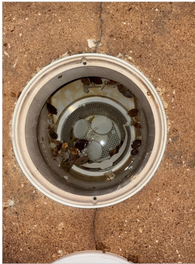
Chemical tablets inside skimmer. The heater manufacturer recommends not to place any tablets inside the skimmers.
