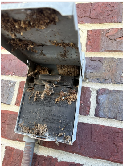
Pest intrusion into HVAC 1 disconnect.
