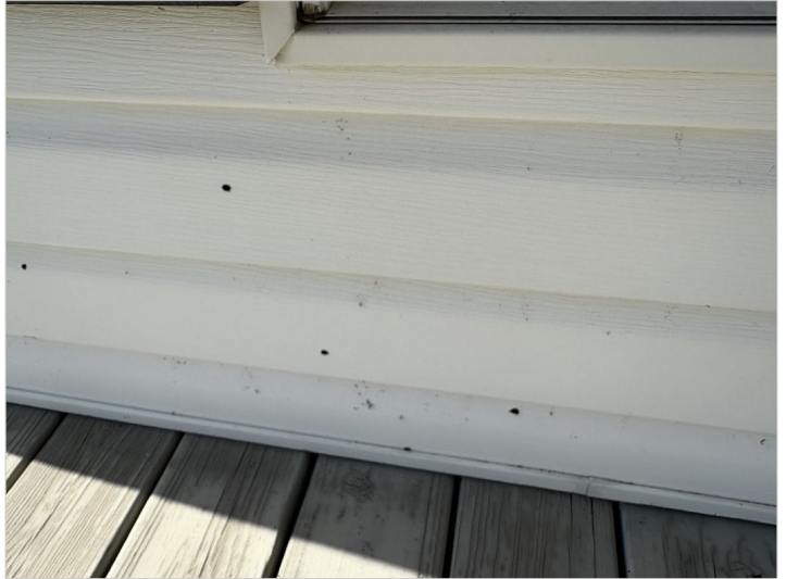
Small holes observed in vinyl siding above front deck.
