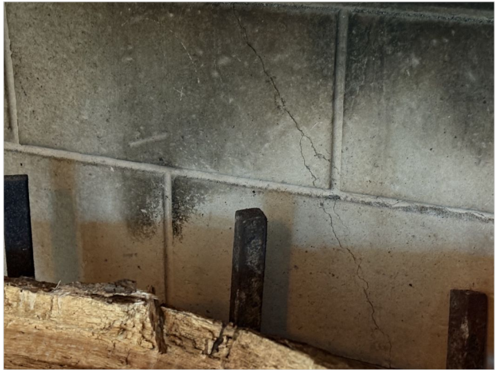
Crack was observed in rear side of fireplace.
