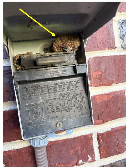
Pest intrusion into HVAC 2 disconnect.
