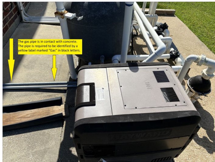
Gas line was in contact with concrete and not labeled properly.
