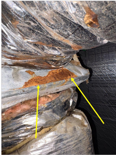
A branch air duct manifold showed signs of moisture damage.
