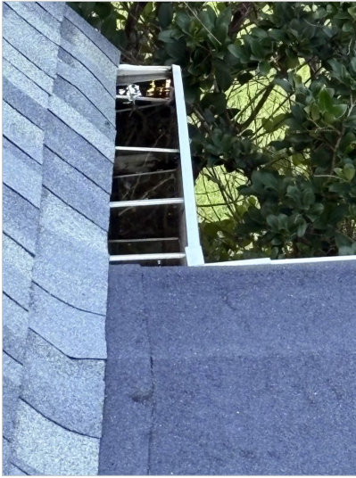
Front right side of home gutters were not draining due to being clogged.
