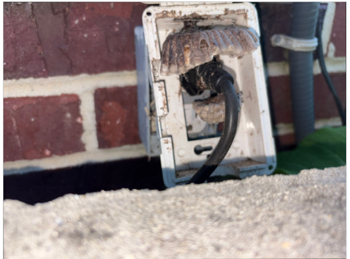
Same receptacle for sewer blower.
