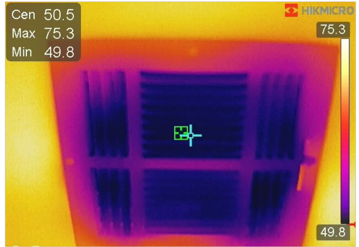
Supply Register Temp: ~ 50°F
