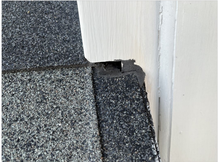
Close-Up of insufficient flashing and sealant located at end of balcony.
