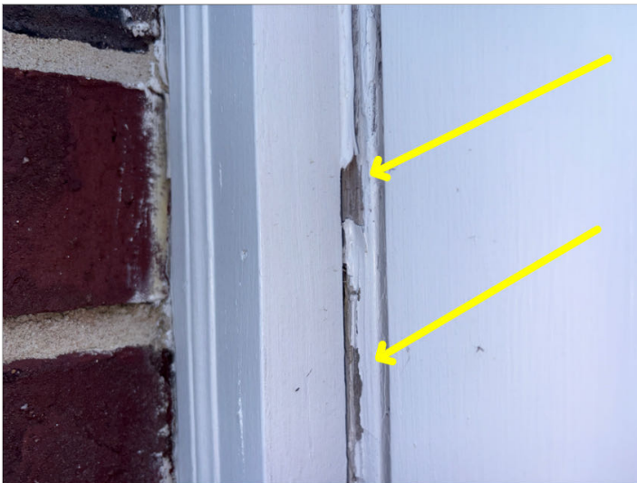
Rear garage entry door frame casing sealant deterioration.
