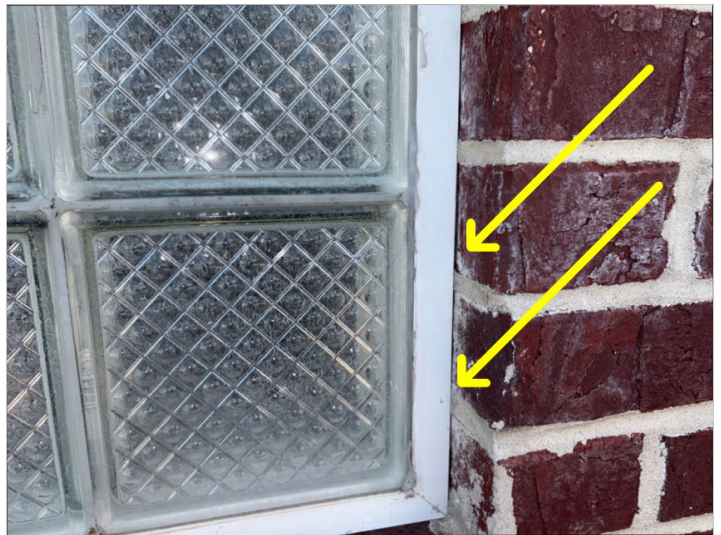
Sealant needed around bathroom window and brick siding.
