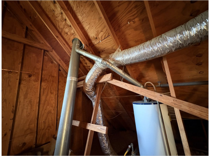
Water heater flue in contact with combustible material. A better option would be for the flue to go straight up to penetrate the roof.
