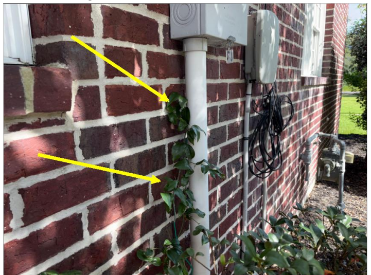
Vine growing toward electrical utility meter.
