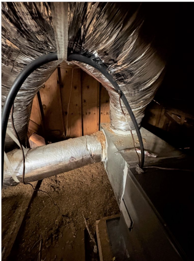
Electrical cable was not properly supported.
