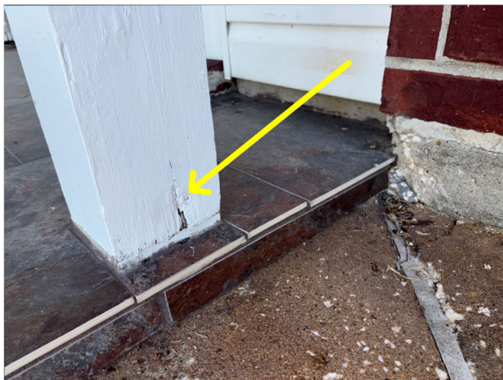
Two of the rear balcony columns were deteriorated.
