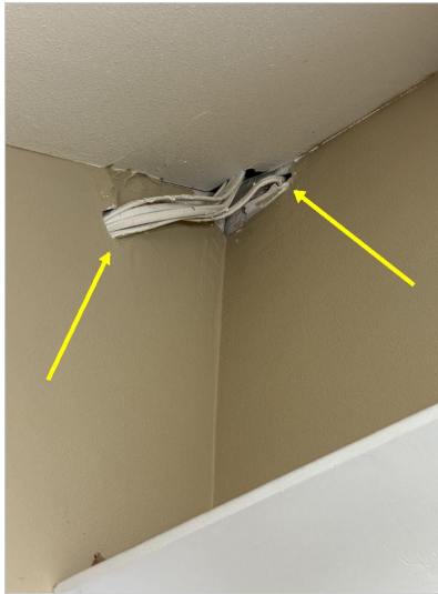
Electrical cables exposed.
