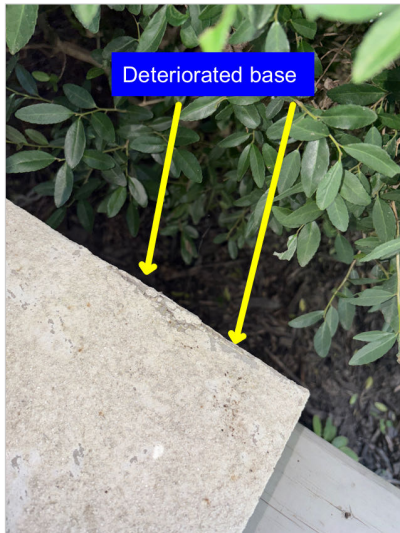
Column base was deteriorated.
