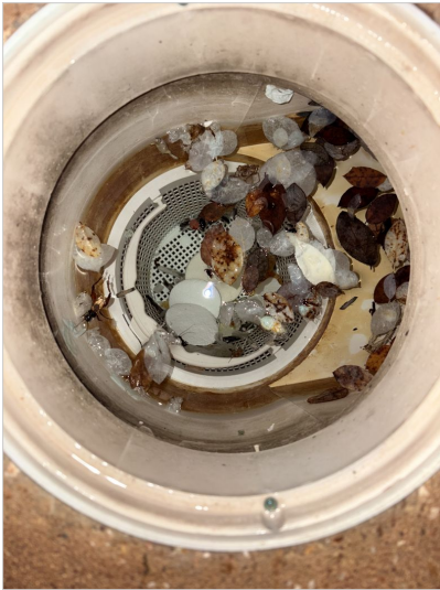
Skimmer is working properly but had debris.
