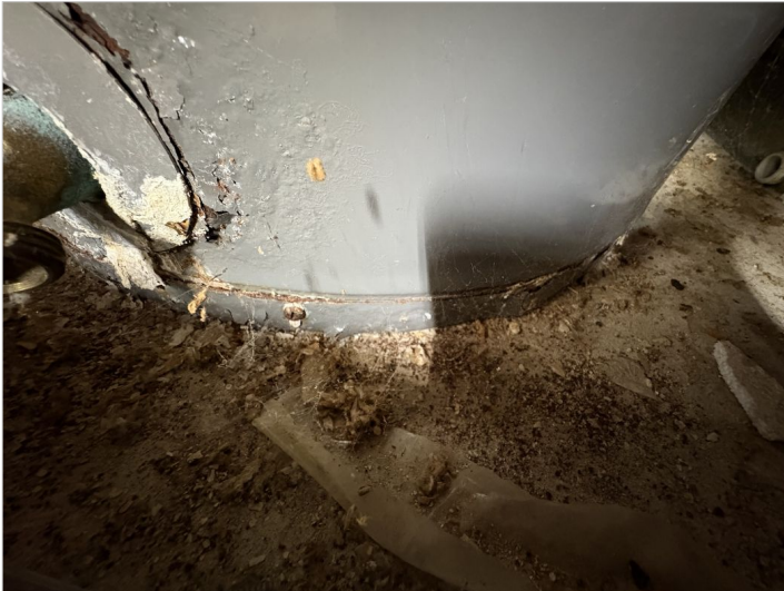
Electric water heater at rear left side of home showed signs of deterioration.
