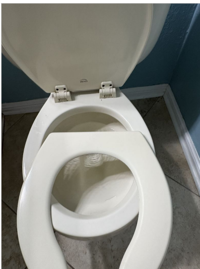
Toilet seat hinges damaged. Located bathroom #4 with double sink.
