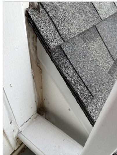
Area of concern for potential water damage located at balcony rail.
